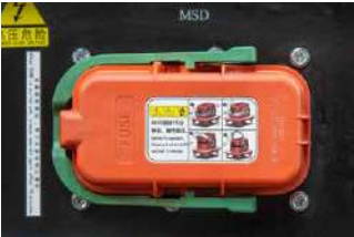
The MSD maintenance switch
